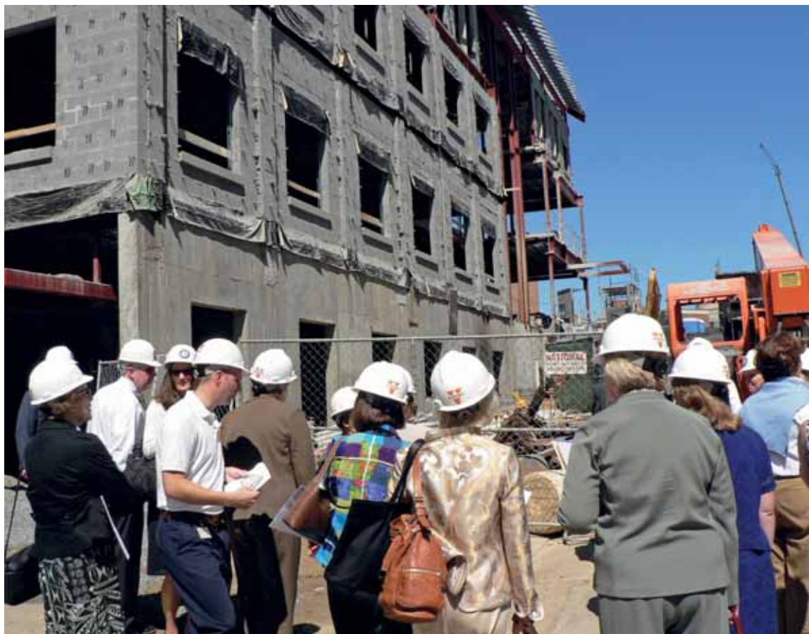
Watching the progress—visitors tour the site of the UVA Claude Moore Nursing Education Building.
